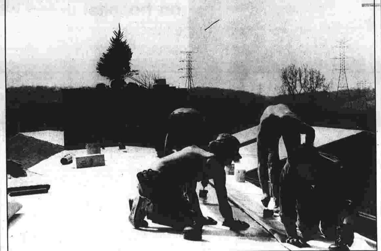
TOPPING OFF — Workers for Midstate Roofing Inc. glue a rubber mat on the roof of the Arbors at Hop Brook, West Center Street, with a "topping-off tree" in the background signaling near-completion of the job. The tree will be planted in front of the building when it is finished. In front are foreman Bob Merkel of Vernon, left, and Rocco Carlini of Manchester. Behind them are Michael Wellington of Vernon, left, and Jim Nesbitt of East Hartford.
